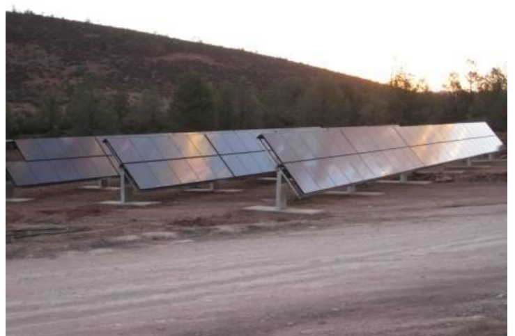
Part of our commitment to the environment we live in, solar panels to power the Eco Villas.
